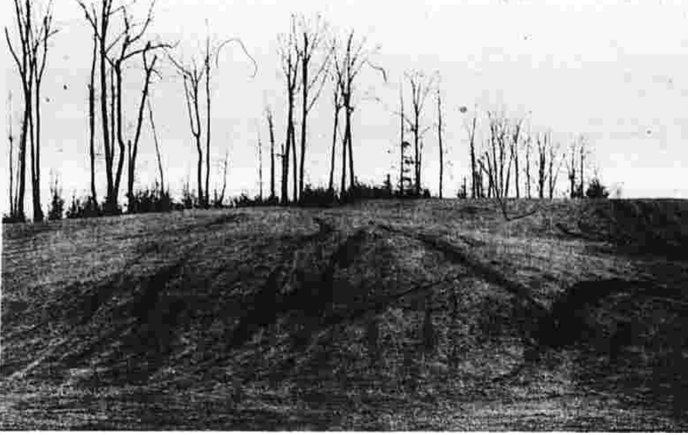
Ski Slope Damage
